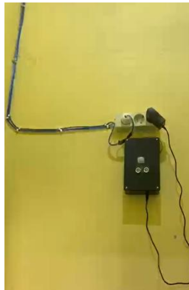
Figure 9. Installation Automatic Lighting
